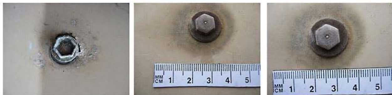
These fasteners are exhibiting corrosion caused by a conductive washer.
