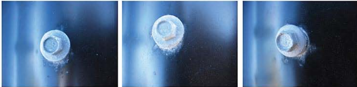
From left to right: Corrosion on colored steel with a mildly conductive washer, semi-conductive washer and highly conductive washer after 10 months exposure.
